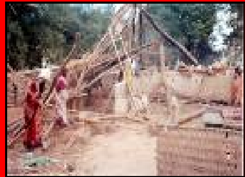
Construction work & debris cleaning as part of Cash for Work activities being conducted in Andhra Pradesh
